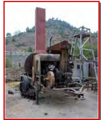
【Photo-41 : Asphalt mixture blender at Hesothangkha factory (Hard to be repaired)】
