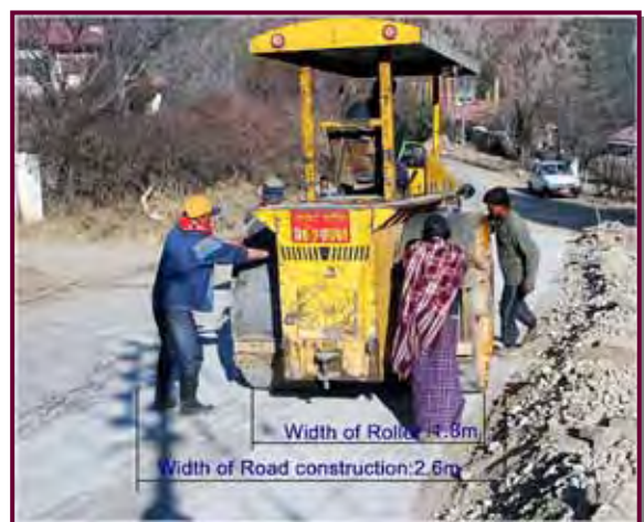
[Photo-36: Too heavy compacting roller]
